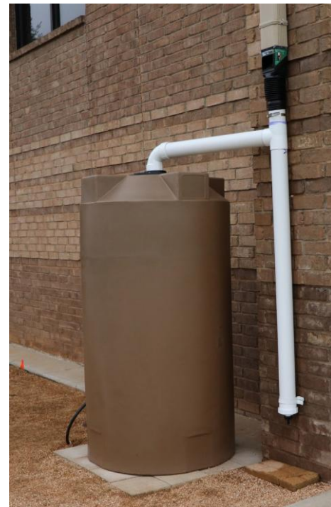
This 300-gallon rainwater harvesting system at the Wolfforth City Library is fitted with a first flush diverter and downspout filter.
